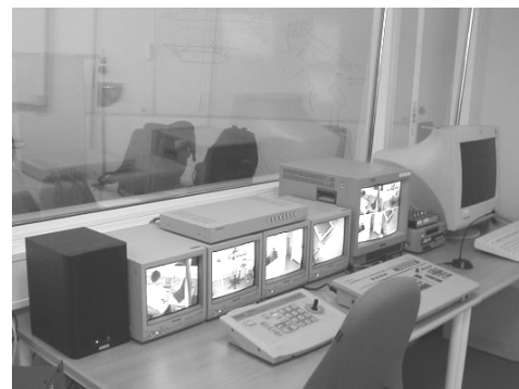
Figure 10. The control room
