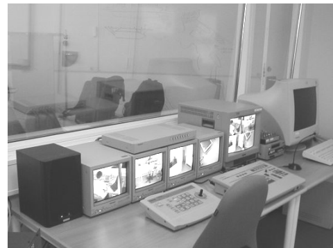
Figure 10. The control room
